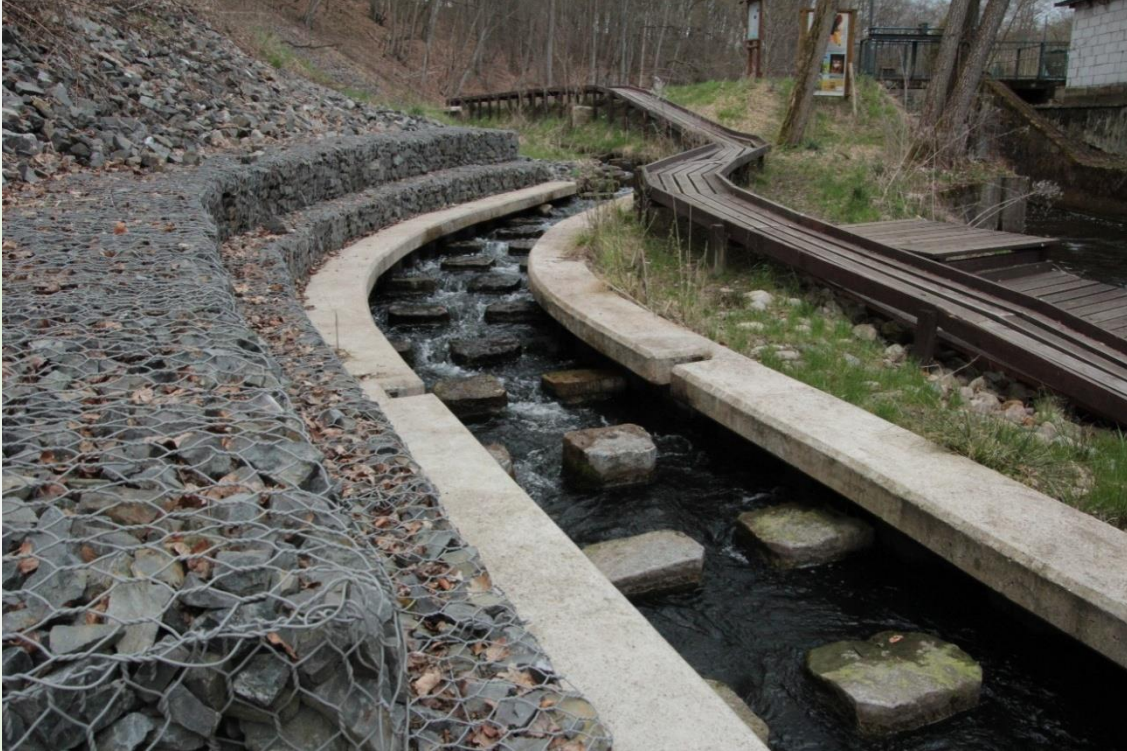
A bottom ramp in the lower section of the Sucha stream built as a protection of the intensely eroding slope of the road embankment for the protection of the only water crowfoot site of proper conservation status in the Drawa National Park.
